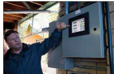
The automated control system allows remote monitoring, control, and data collection using an iPad, iPhone, or computer using a secure internet connection.
