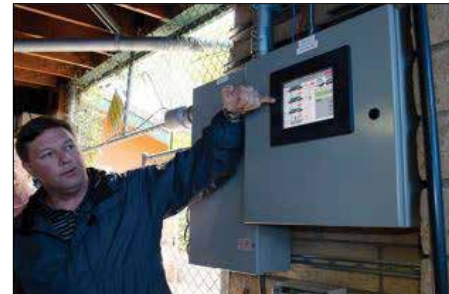
The automated control system allows remote monitoring, control, and data collection using an iPad, iPhone, or computer using a secure internet connection.
