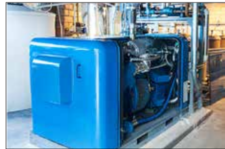
The cogeneration system consists of a 75 kW module installed in the existing pump room, requiring no additional space.
