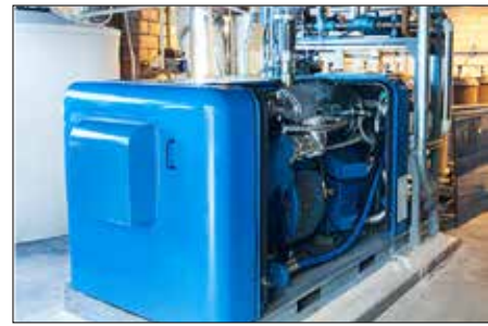
The cogeneration system consists of a 75 kW module installed in the existing pump room, requiring no additional space.
